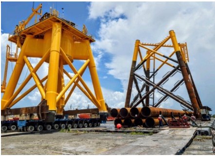
Jacket foundations for the Block Island Wind Farm, designed by Keystone Engineering. Credit: Keystone Engineering
